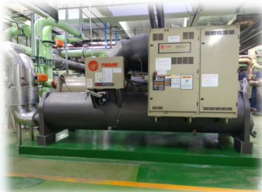
▲ Inverter Type Centrifugal-chiller
