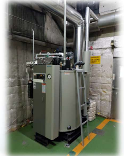
▲ High efficiency Steam Boiler
