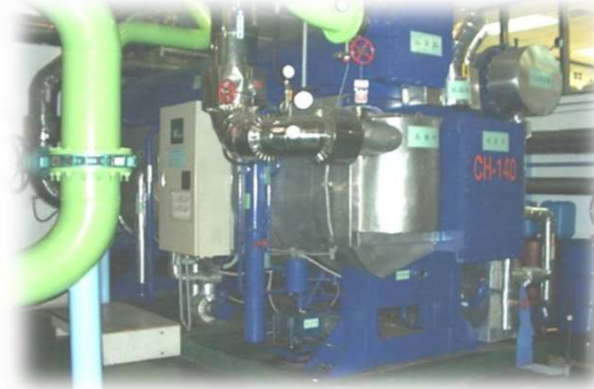
▲ Steam-fired Absorption Chiller
