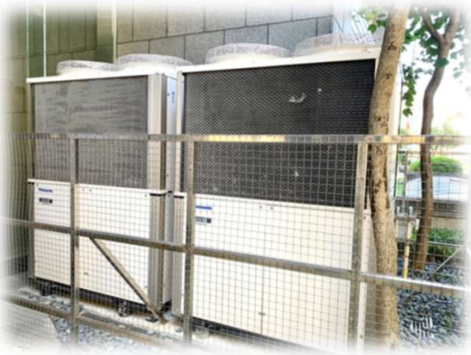
▲ GHP Gas-driven Air-conditioner
